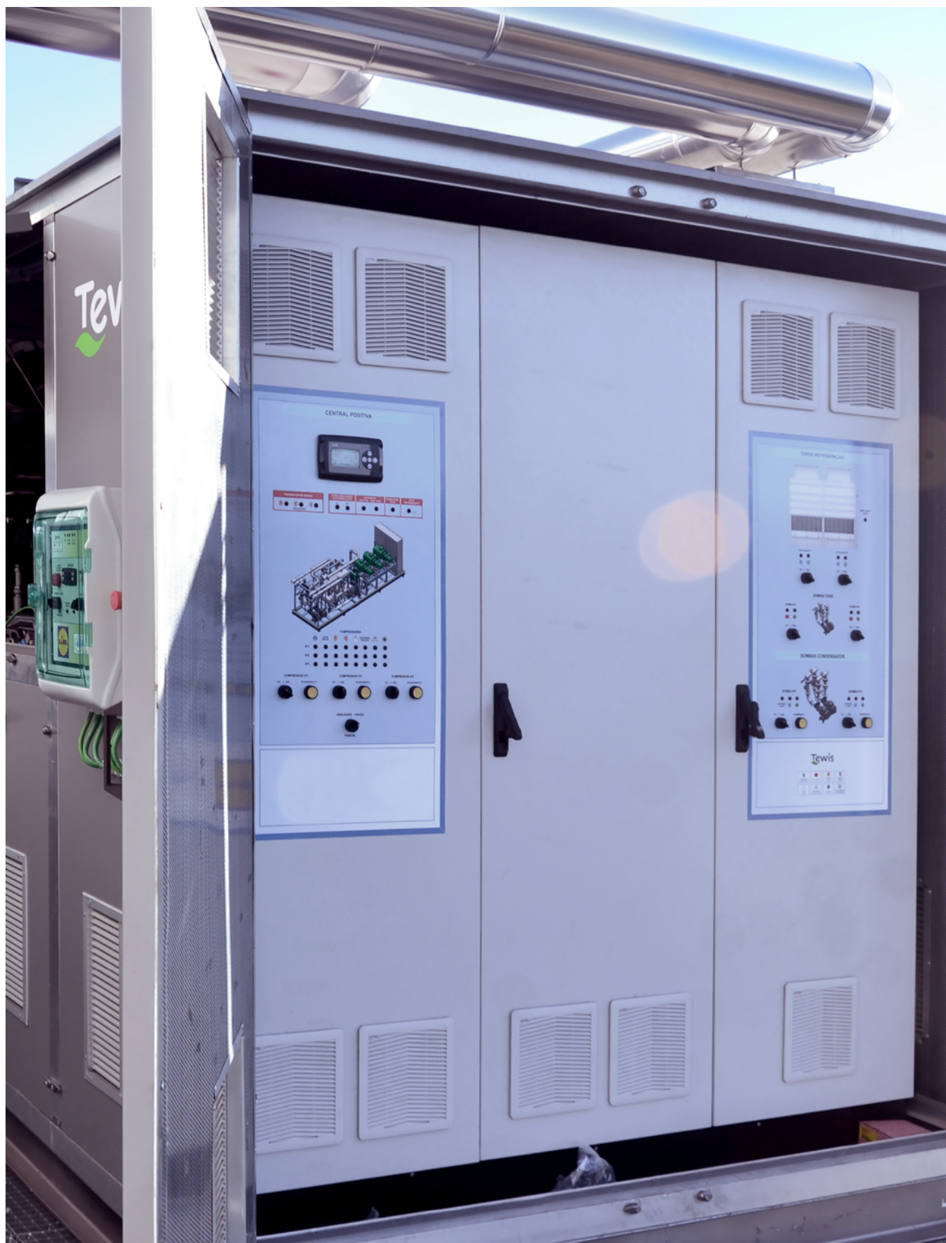
Multi-compressor packs and racks
