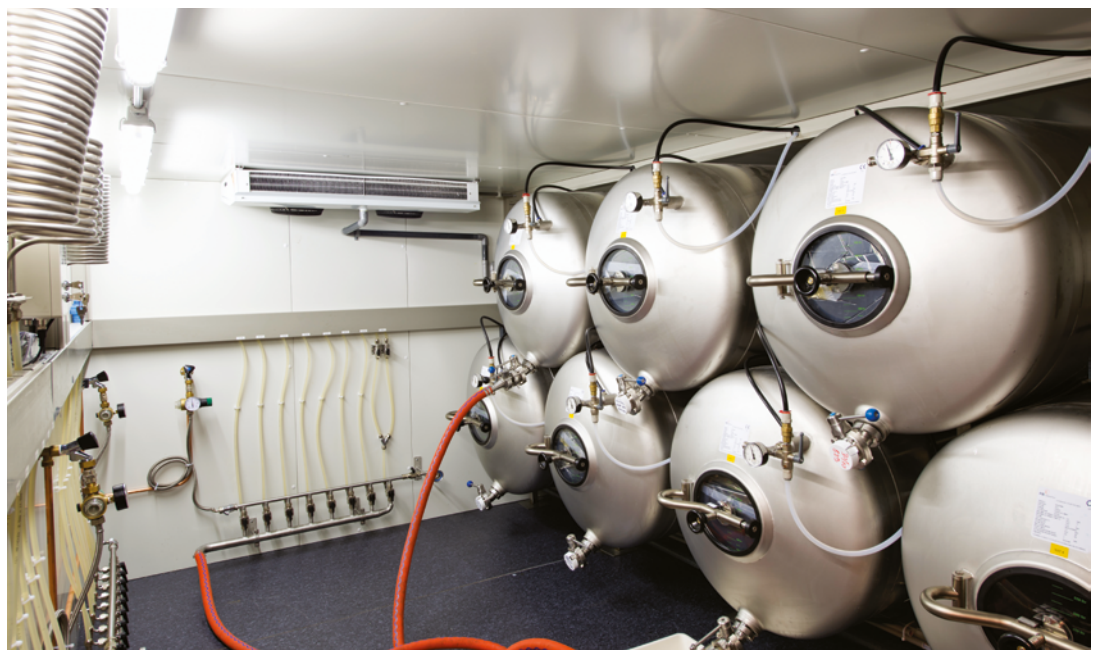
Beer cooling facility, chilled with ZEAS
